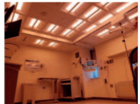
Installed in a hospital
